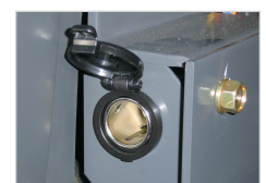
Backup Power Supply
